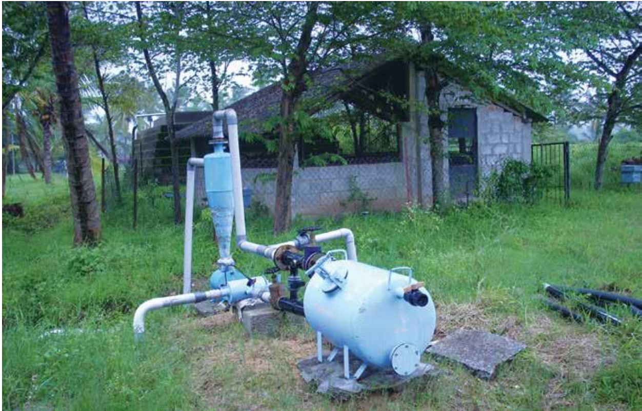
Figure 2.3. Head control unit of drip irrigation
